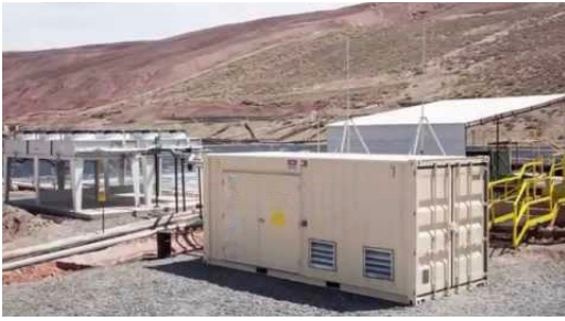
Figure 5 ORC Site with Air Cooling
